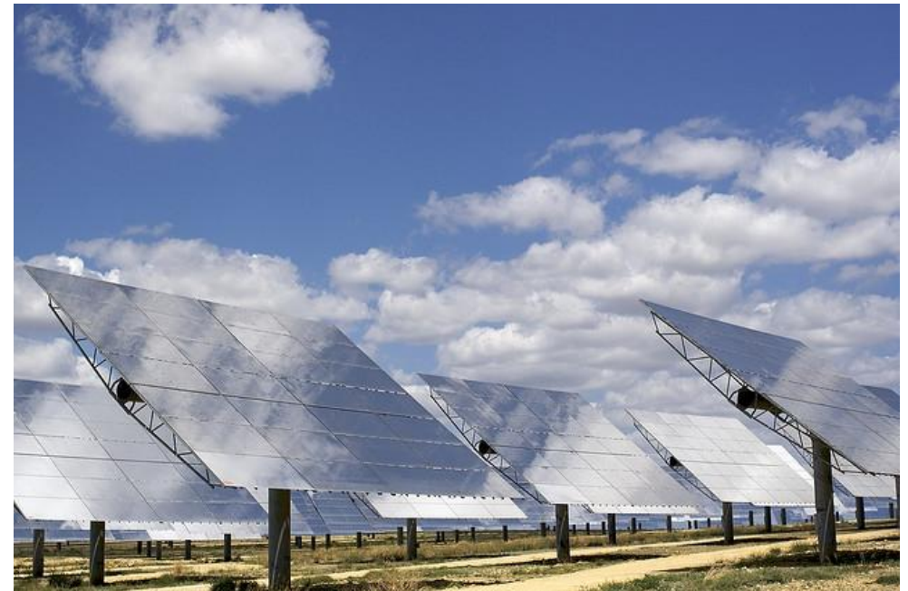
Mirrors from a Concentrated Solar Thermal power plant. Source: langalex on Flickr.com
